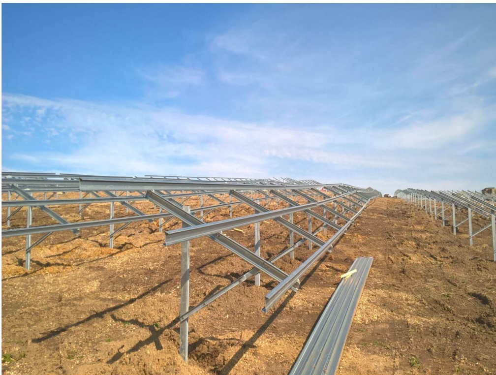
Schletter racking system.
